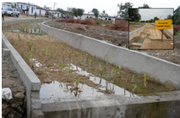
Constructed wetland at Kothapally village in India. Treated water being used to irrigate one hectare farmland.
